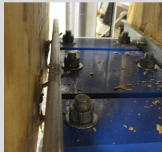
Figure C-1 Photograph of Clamping System
